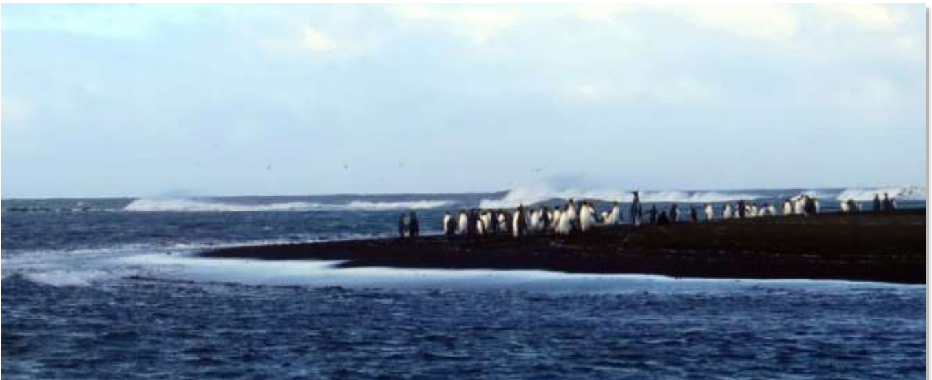
Figure 150 – The west side of the south entrance. Clearly, the original breakwater is almost totally reduced to wash rocks.
